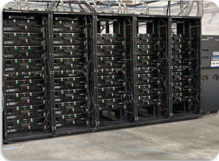
Fit to Existing Racks
